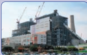
Linkou Power Plant, Taiwan, where MHPS has been testing the new combustion control technology
