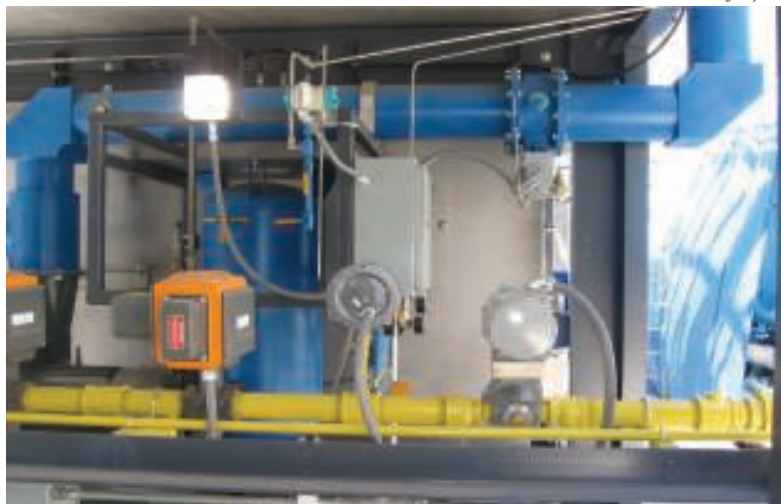
FIGURE 4. The Air Gas Ratio Control (AGRC) system measures and controls gas and air flows continuously through a PID loop to provide less energy use and lower emissions rates
