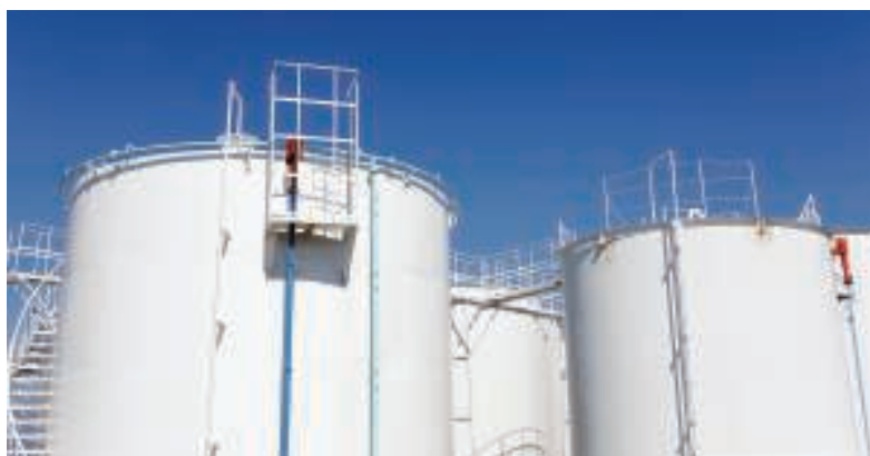
FIGURE 1. Storage tanks are a common sight at petroleum refineries and petrochemical plants
